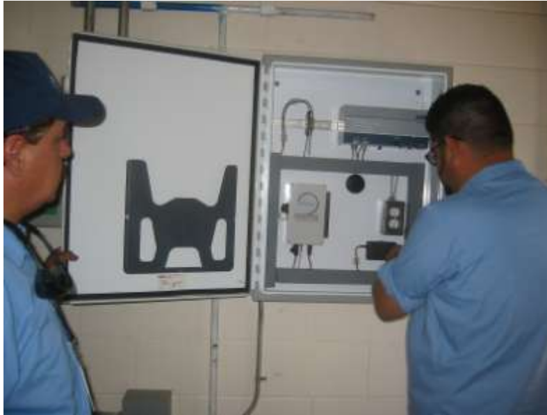
Figure 3 – TP1 Transient Pressure Monitoring System Installation
